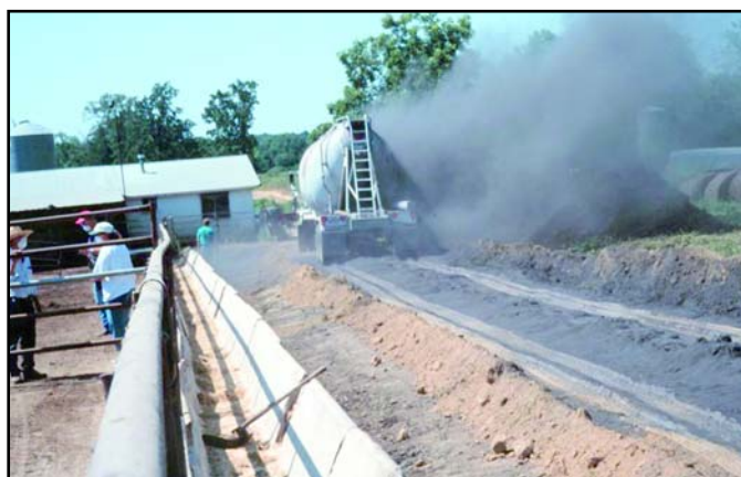
Fly ash being delivered to the farm where it will be mixed with clay soil prior to watering and placement. The mixing area is an existing road surface with the clean clay material for mixing windrowed on each side of the road.
